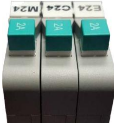
Figure 75: Breakers in the OFF Position
