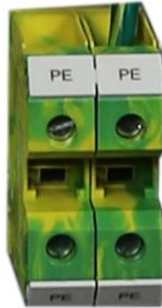
Figure 6: Ground Bus Terminal Blocks
