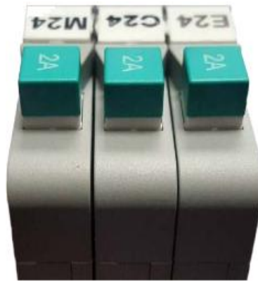
Figure 115: Breakers in the OFF Position
