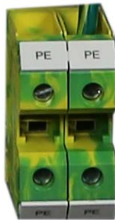
Figure 6: Ground Bus Terminal Blocks
