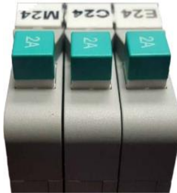
Figure 75: Breakers in the OFF Position
