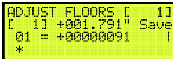
Figure 231: ADJUST FLOORS Menu – Too Low
