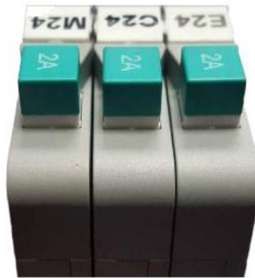
Figure 115: Breakers in the OFF Position
