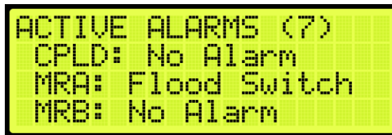
Figure 758: Active Alarms Menu
