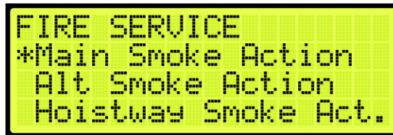
Figure 565: FIRE SERVICE Menu – Main Smoke Action
